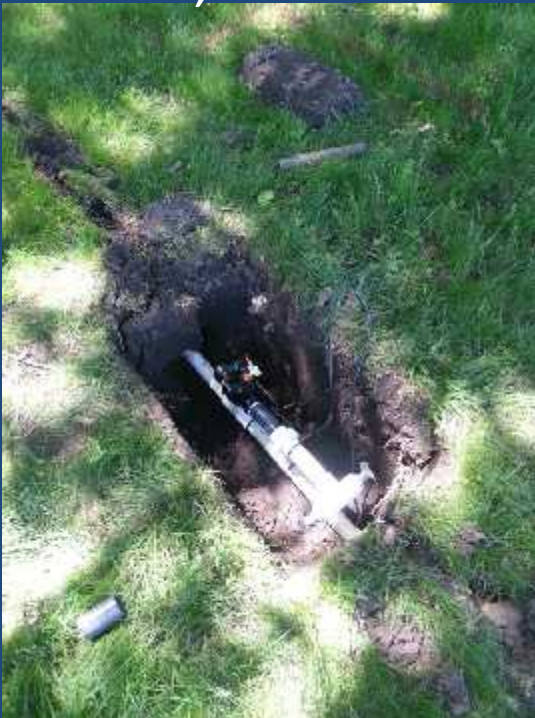
New Valve Box at Upper Park
