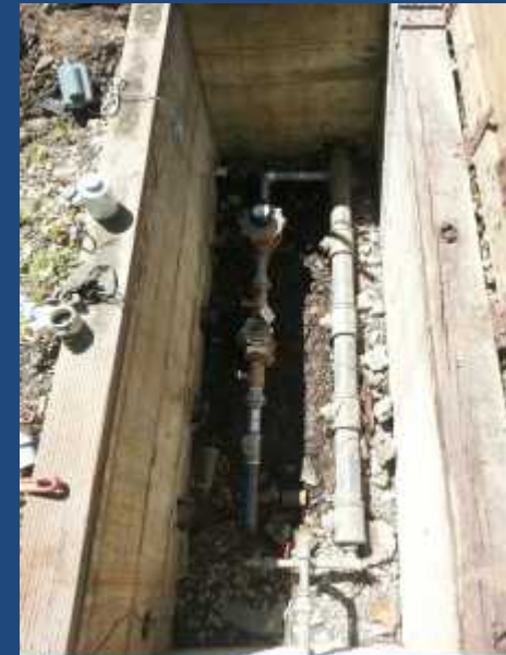
Old Valve Box at Memorial Park
