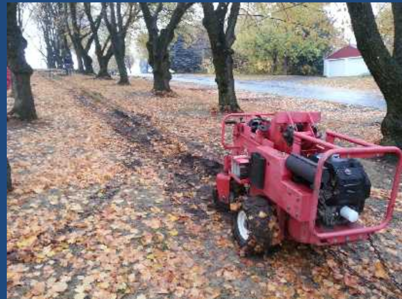
Sprinkler Head location Moved Inside Tree Line
