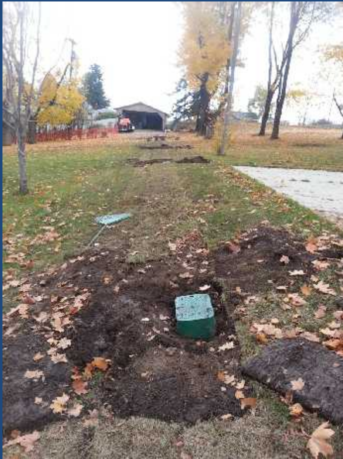
New Valve Box at Upper Park
