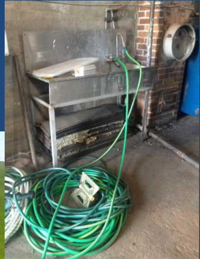
Irrigation system before
