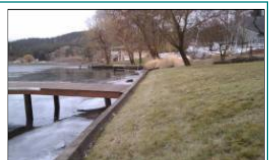
The failing bulkhead prior to removal
