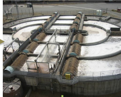
Orbal Activated Sludge
