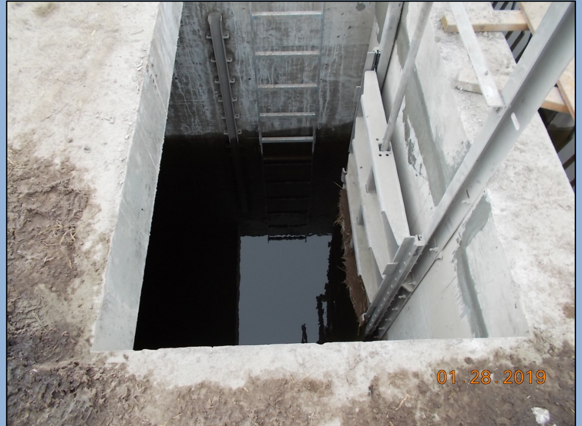
Interior of outlet control structure, including head gate and rails for elevation control boards
